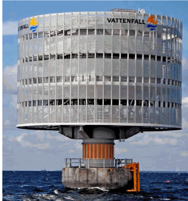
Figure 72 – The offshore substation installed at Lillgrund [373]
