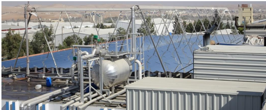
Fig. 1: Collector Field and Steam Drum on the RAM Pharma Rooftop
