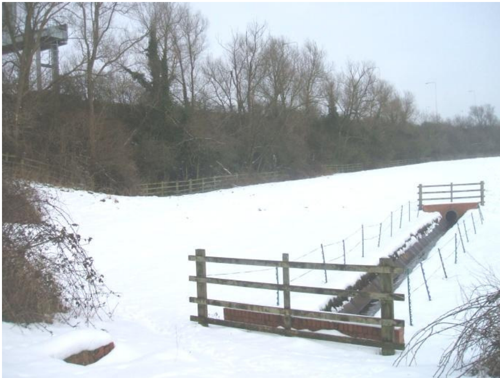
Fig. S1e. Motorway runoff discharge pipe just prior to discharge to Battlefield Brook just upstream of Site 4 (M5 is in the background).
