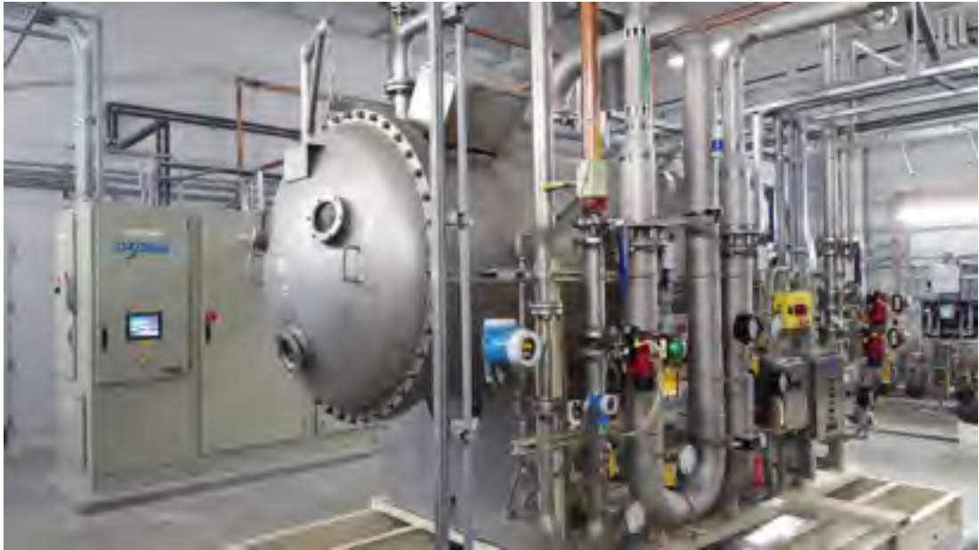
Figure 6.4 A 400kW ozone generator and its PSU in the background, where we can see in the foreground the process piping, valves, and various meters used to control the gas and the cooling water flowing into the generator vessel
