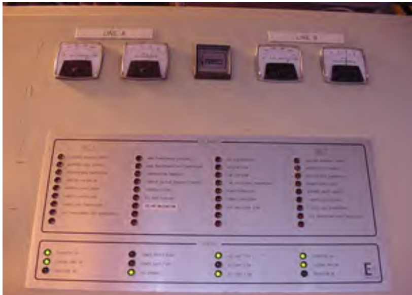
Figure 6.7 Door-mounted alarm annunciator and analog meters
