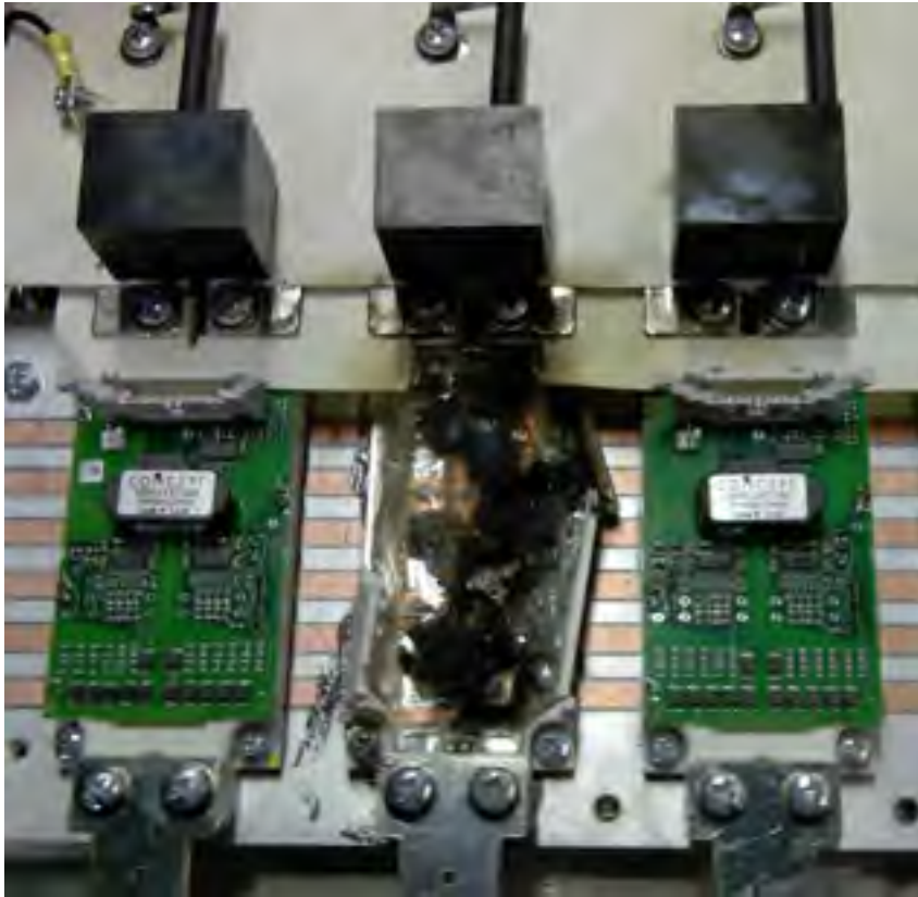
Figure 3.21 IGBT damaged by an explosion
