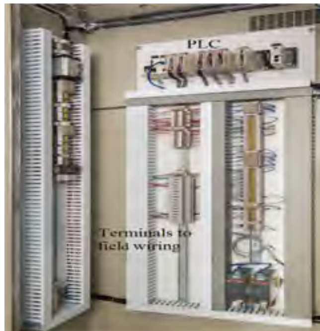
Figure 3.3 Industrial control panel with PLC and field terminals
