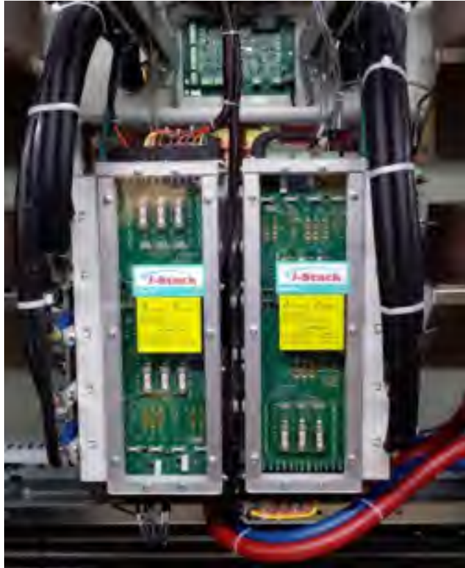
Figure 3.26 Two I-Stacks mounted in a cabinet with auxiliary components
