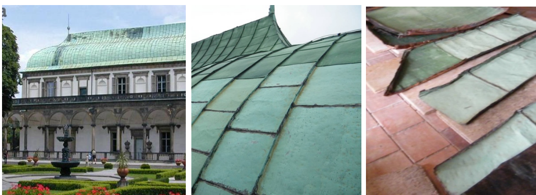
Figure 17: Copper with a natural patina was obtained from the roof of Queen Anna's Summer Palace in Prague (Kreislva & Geiplova, 2016; Kreislva & Koukalová, 2012)
