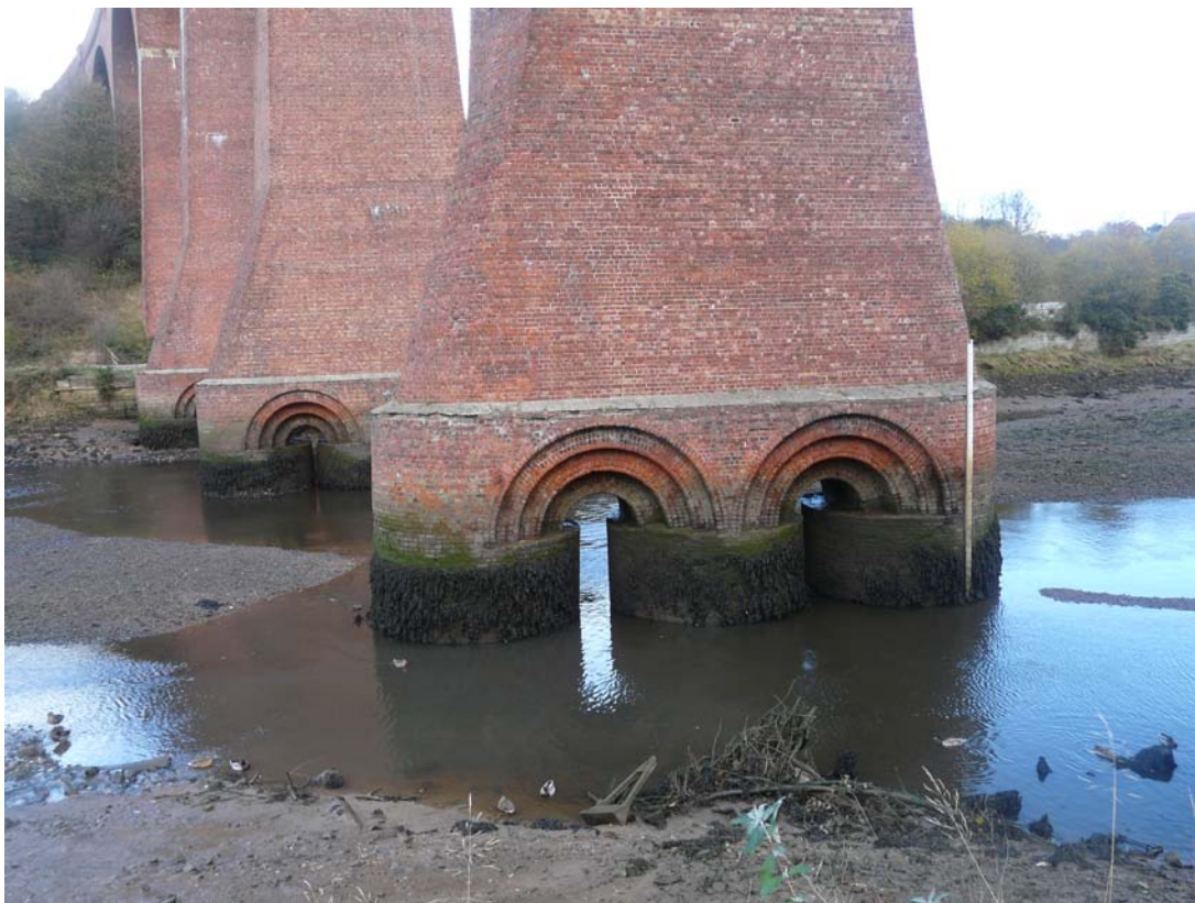
Figure 2. A view of the caissons and arches of the foundations for Pier 5
