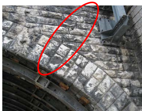
Figure 3-2 Renforcement et fissures.
