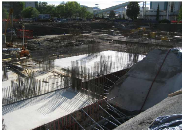
Slika 2.16: Gradnja temeljev glavnega tehnološkega objekta šestega bloka v termoelektrarni Šoštanj. Figure 2.16: Construction of foundations of main power facility of the 6 th unit at Šoštanj power plant.
