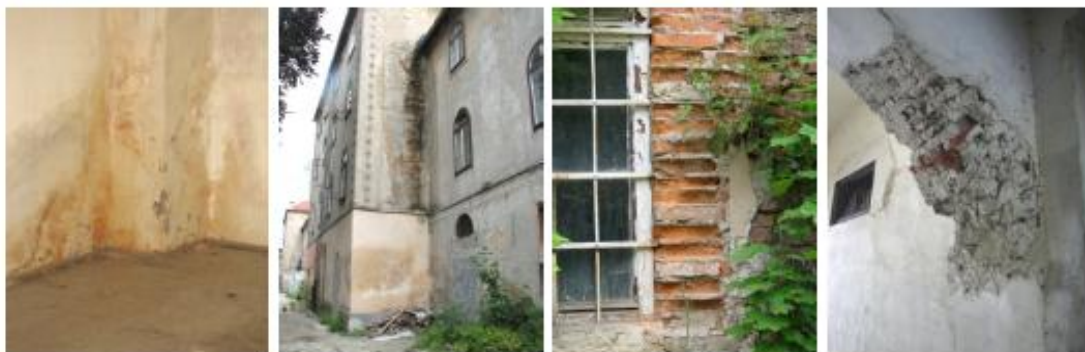
Figure 2. Deterioration due to capillary rise, inadequate drainage, freezing-thawing and overloading
