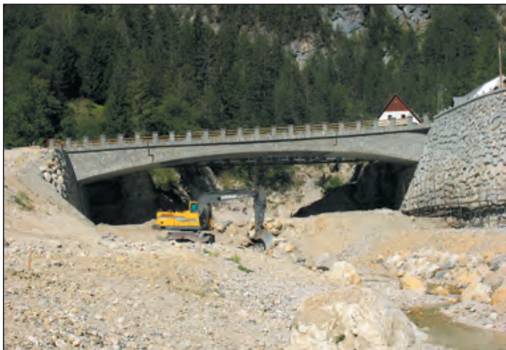
Figure 6: A view of a new reinforced concrete road bridge in Gorenji Log on September 9, 2006 (upstream view, compare the executed bridge with the preliminary design on Figure 5).
