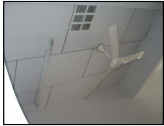
Figure 4: Vents and Fan Location in the Experimental House
