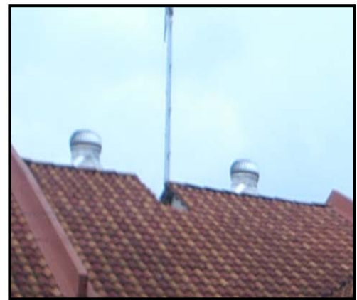
Figure 2: Ventilator Location at the Top of Experimental House Roof
