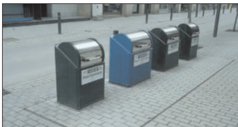
Picture 015 > Buried container with accessible mouth Solutions should be designed to allow everybody to participate in the recycling process
