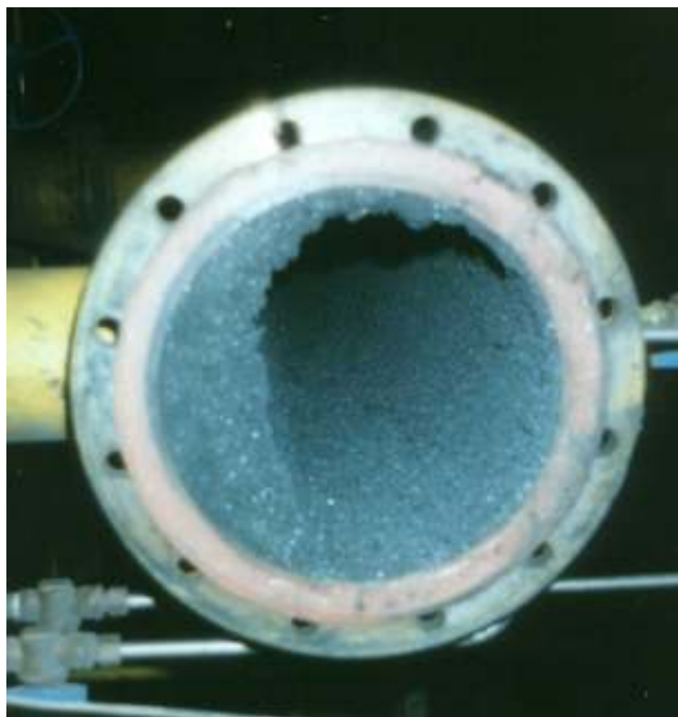
Figure 1. Photo of the contaminant material deposited from the process gas onto the wall of a pipeline.
