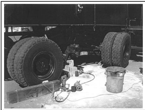
Fig. 1 General view of two crane wheel sets and one failed axle (middle) with wheel and wheel hub removed. The wheels are turned at different angles.
