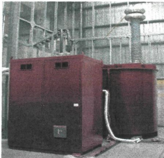
Figure 3-7. 350 kV/700kVA AC high voltage system
