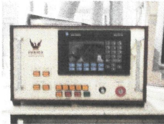
Figure 3-8. Control unit for 350 kV Transformer.
