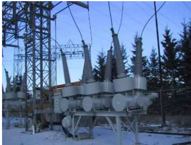
Figure 2.3: Dead tank circuit-breaker (Source: Manitoba, Canada)
