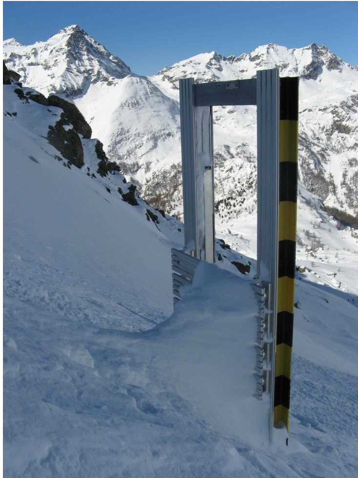
Figure 4: View of the obstacle after an avalanche event. Only the upper part of the steel structure emerges from the snowpack.
