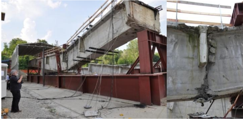
Figure 22 B04: views of collapsed beam
