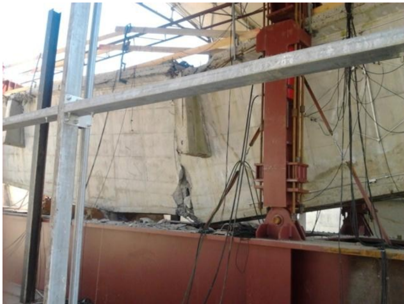
Figure 13 The beam collapsed after static test
