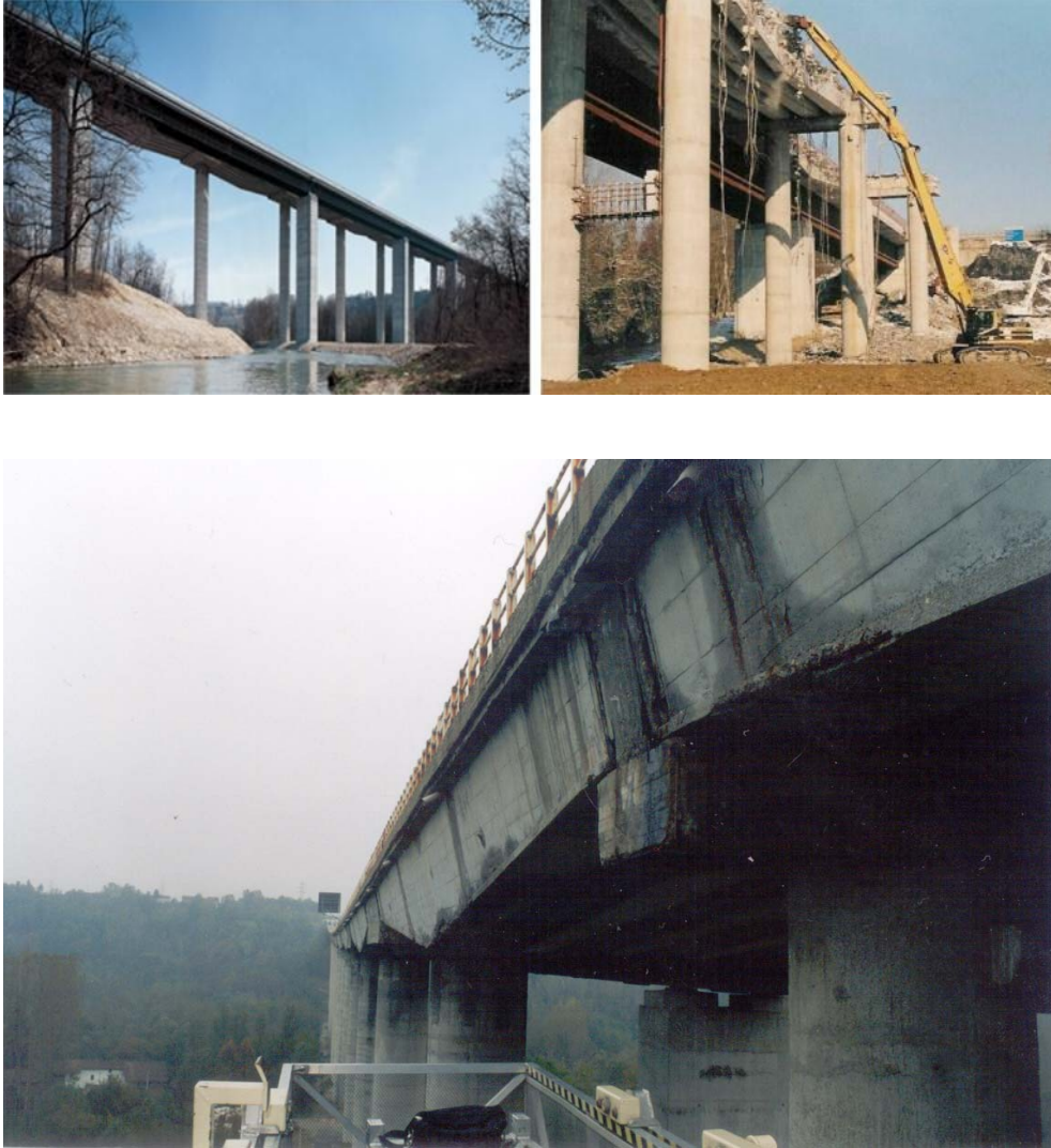
Figure 1 Views of the Pesio viaduct and a phase of the demolition of the decks
