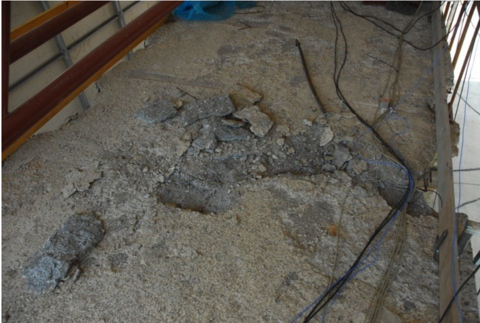
Figure 17 View of the failure section on the upper slab
