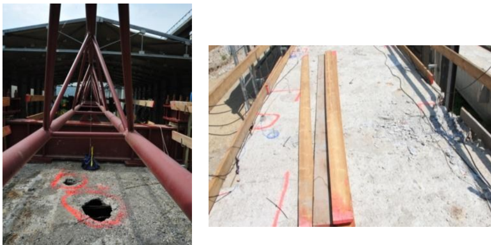
Figure 39 B07: localized damages on the slab and a view of the failure section
