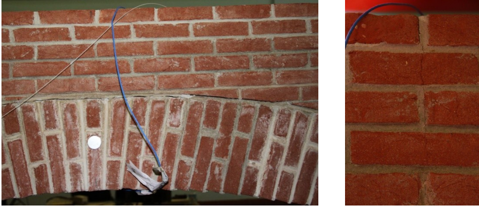
Figure 7 Crack pattern after damage step 9
