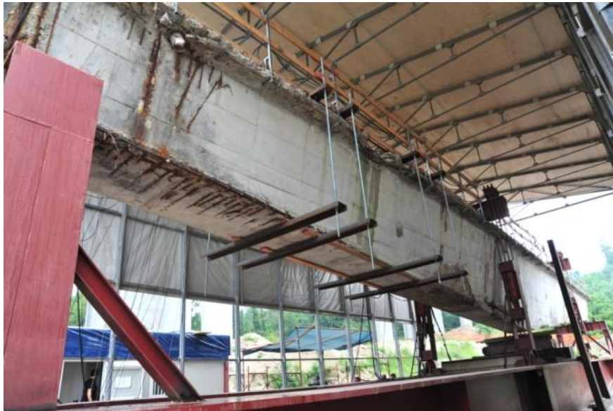
Figure 36 Beam B07: view of the beam on the bench test (east side, the most degraded)
