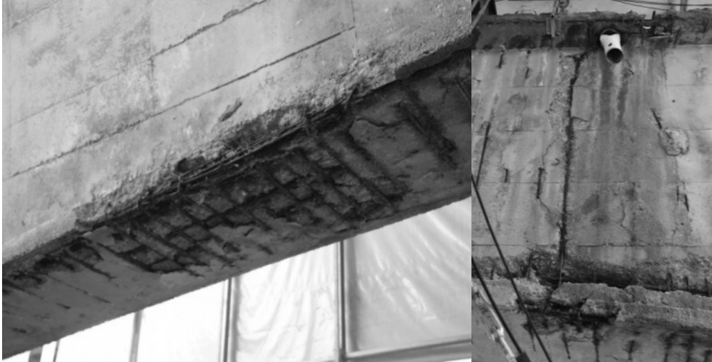
Figure 47 Beam B07: corrosion of the post-tensioned tendons and ordinary reinforcement. The deterioration is particularly advanced in the sections next to the drainpipes
