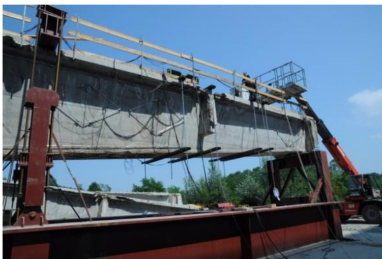
Figure 8 View of the vibrodyne anchorage system
