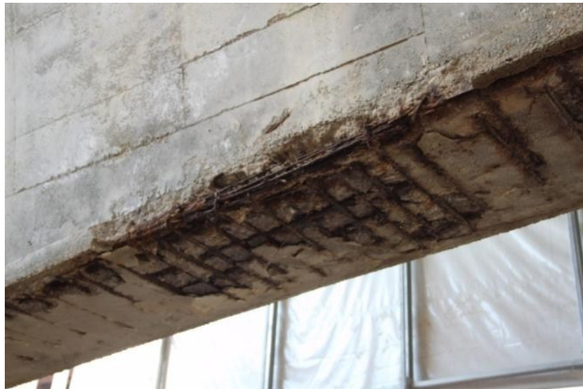
Figure 37 East side of B07: corroded ordinary reinforcement and tendons
