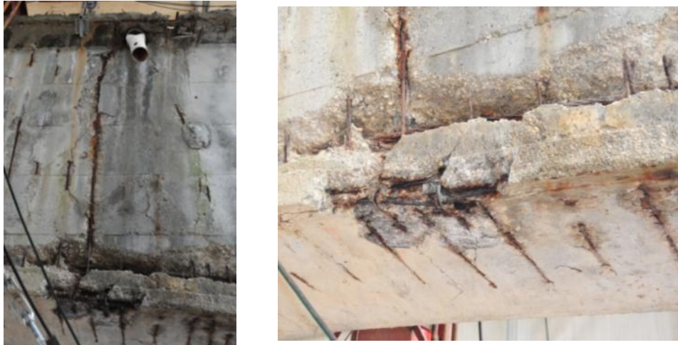
Figure 38 B07: post-tensioned and ordinary reinforcements corroded (east side)
