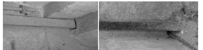
Fig. 11. Pictures of two iron chains from the Amiens Cathedral in France. The left chain appears well preserved while the right chain shows corrosion in evolution. Both chains are in their original state, as installed in the fourteen century, without any protective coating. The distribution of the corroded chains does not follow a specific scheme.
