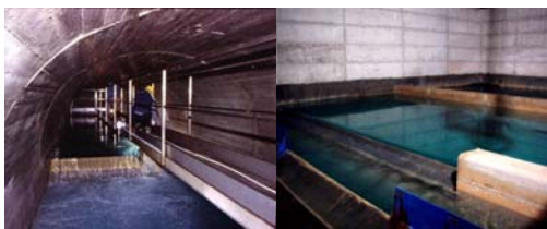
Fig. 7: On the left: the current tapping works; on the right: surge tank of aqueduct
