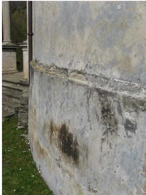
Figure 2. Detachment of historical exterior plasters at Transfiguration Chapel because of the rising damp effects due to capillary action or rain infiltration
