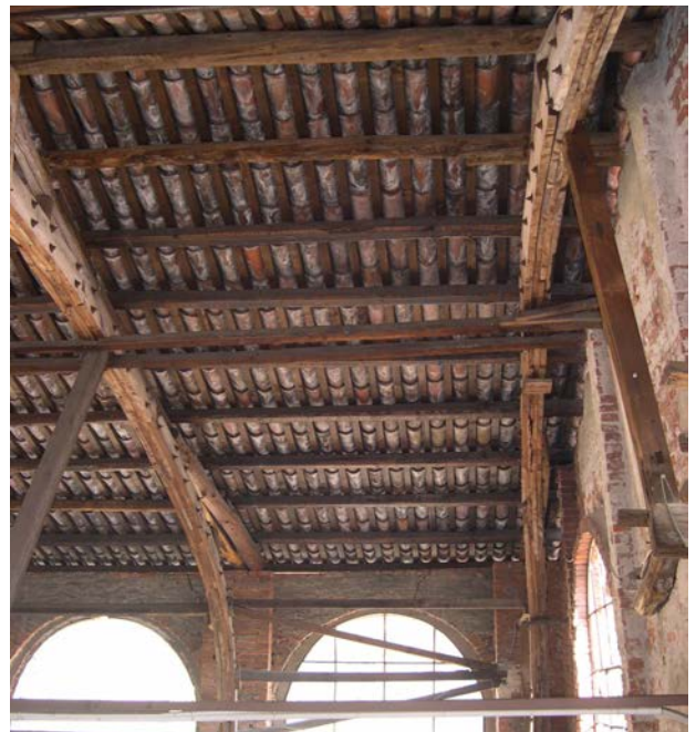
Figure 6 – The former Trombetta wool mill, Biella. Detail of the unstable arches. (photo Mattone).
