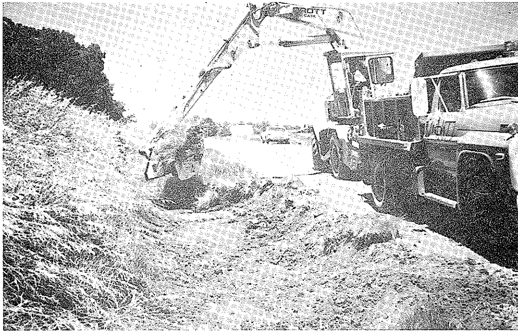
Figure 16. Ditch cleaning operations leave bare soil exposed for invasion by weeds.
