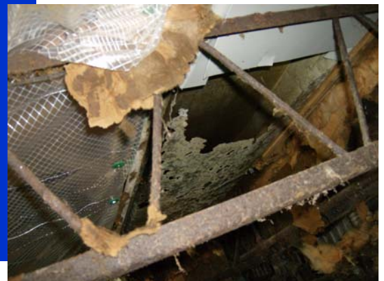
Hmmm...Do you think this duct works?
