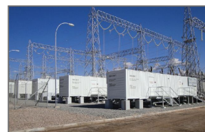
Dynamic energy solutions for a smarter grid
