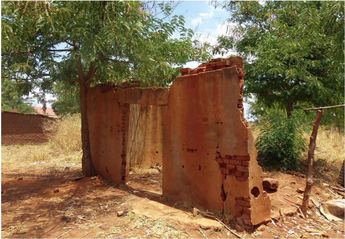
Fig. 8: Remnants of building in Lagi Boma destroyed during the SPLA attack in 1989, February 2014
