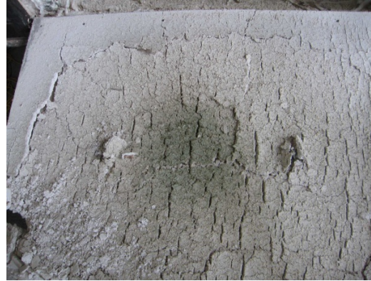
(b) Glass Fibre Insulation is totally burnt Leaving a Dark Stain Behind
