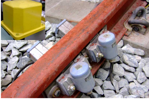
Fig. 2. Axle counter consists of two pairs of transmitter and receiver. Inset shows the track side converter equipment connecting the axle counter.
