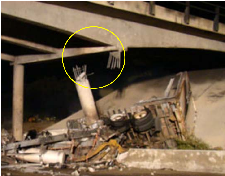
Figure19: Damaged column under vehicle impact
