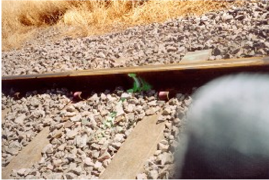
Figure 3.8 HTT Weld Classifications – Not within Tolerance
