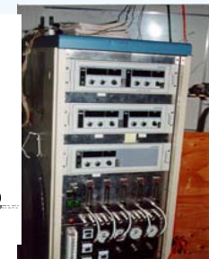
Industry Standard Continuous Emission Monitoring Equipment
