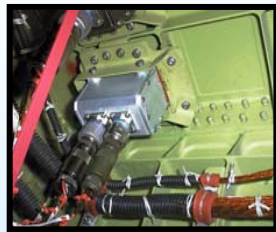
Aft Compartment Hydrogen Monitoring
