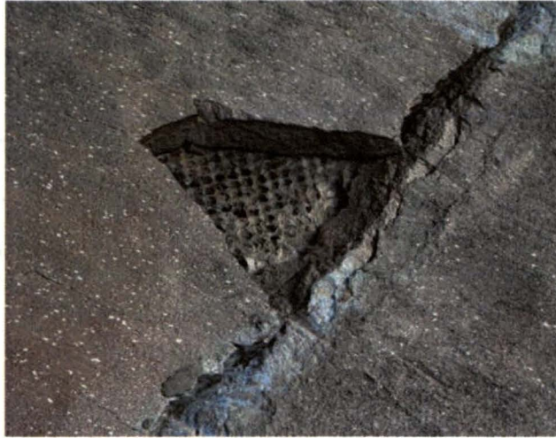
Figure 6. STS-126 Spalled and Dislodged Concrete Section
