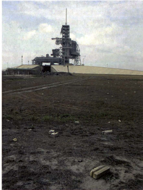
Figure 10. Refractory Concrete Bricks Torn Away From the Flame Trench
