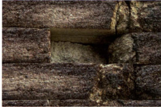
Figure 8. Missing Refractory Brick at LC 39A
