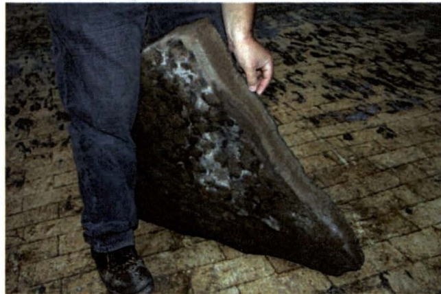
Figure 7. Section of Refractory Concrete Dislodged During the Launch of STS-126
