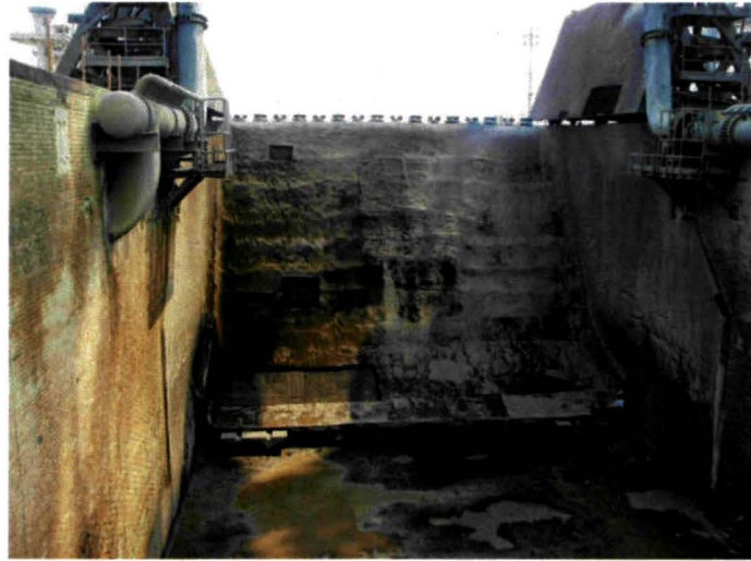
Figure 1. Degradation to Fondu Fyre on the SRB Flame Deflector
