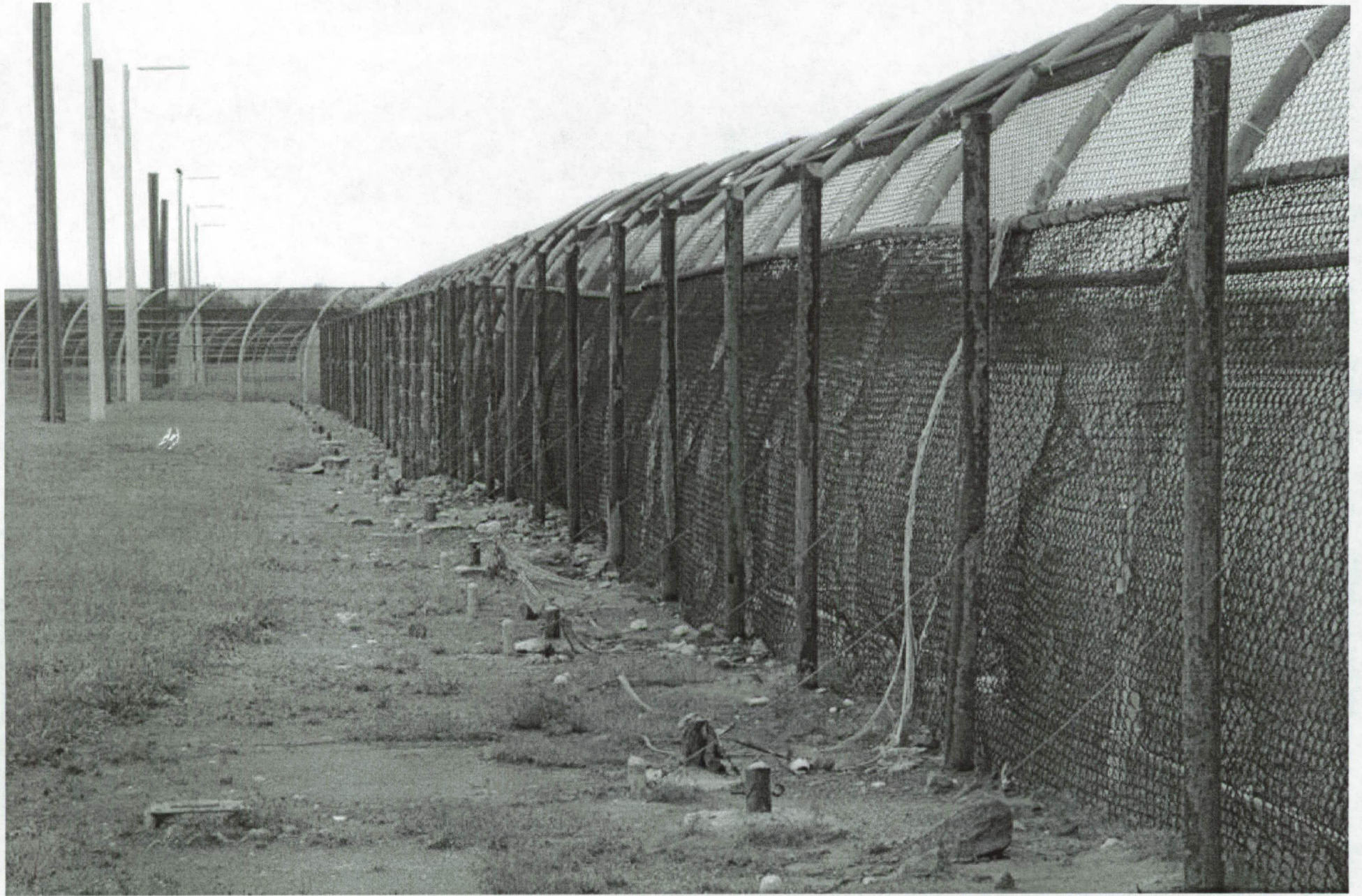
Damage to Pad perimeter fence from chunks of martite blown out of the flame trench
