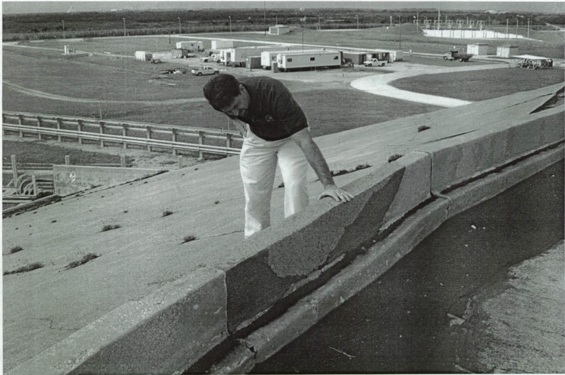
Damage to concrete wall due to FOD caught in the launch blast
