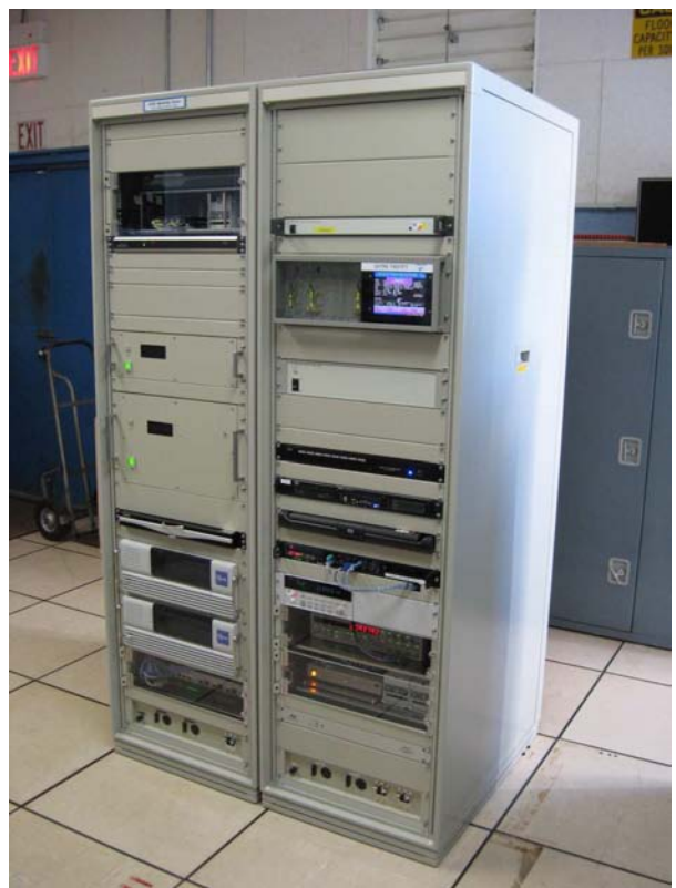
Figure 4. QZSS/TWSTFT equipment racks.
