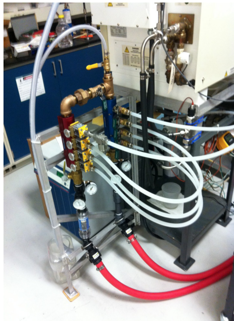
Figure 6. General purpose water-cooling manifolds.
