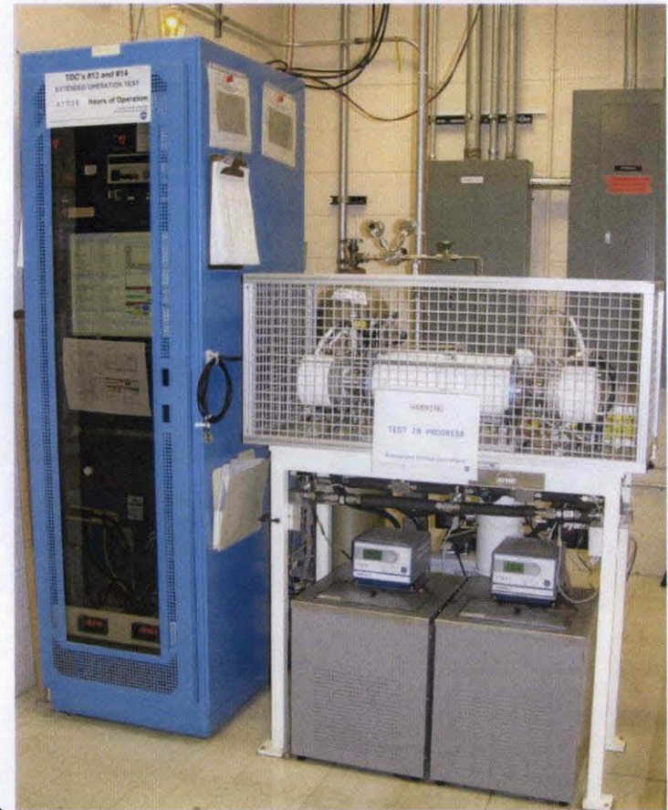
TDC #13 & #14 test station
