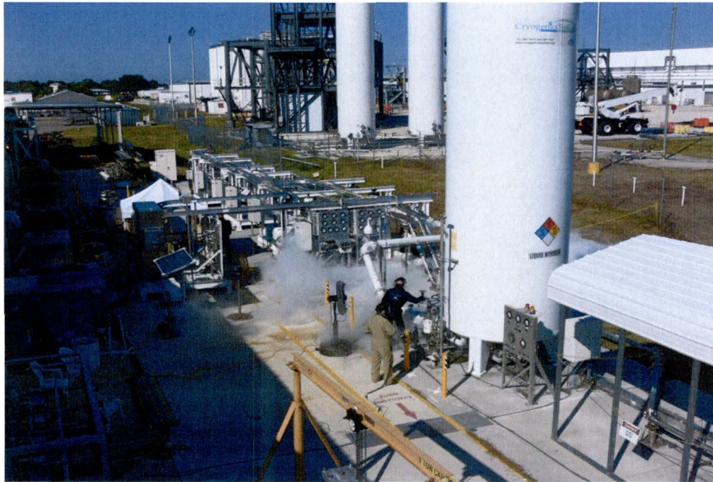
Figure 2-1. The GODU Autonomous Control unit at the KSC Cryogenics Test Laboratory
