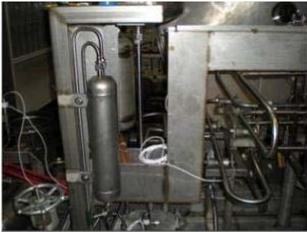
Cable tray providing protection from heat/NaK
