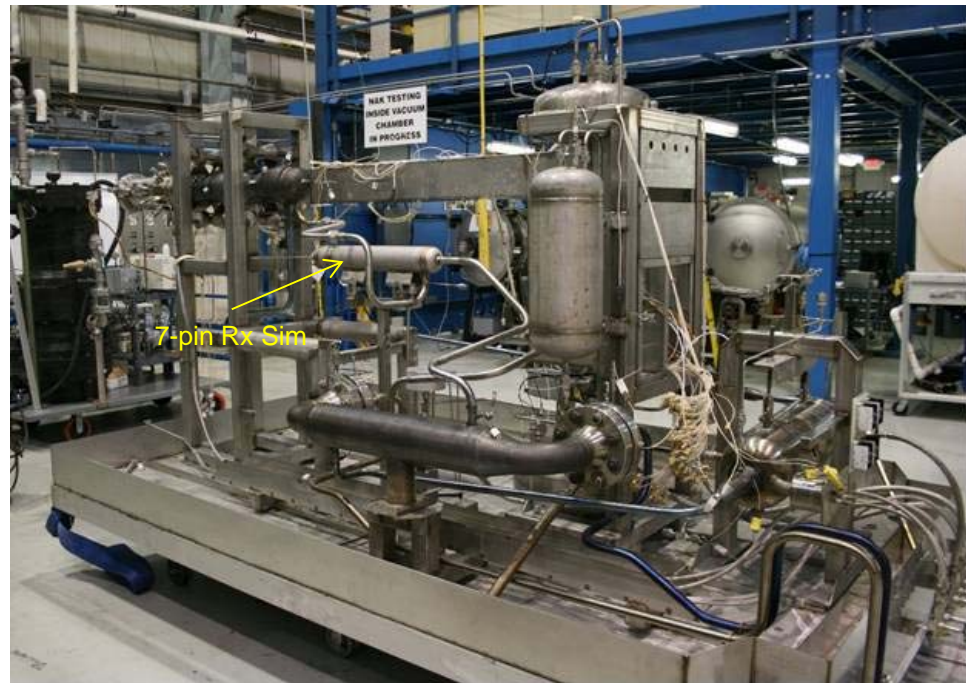
7 Pin Rx Core Sim installed in FPS-PTC
