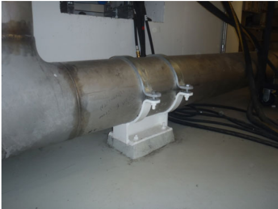
12 inch Riser Floor Pipe Support (PS-1)
