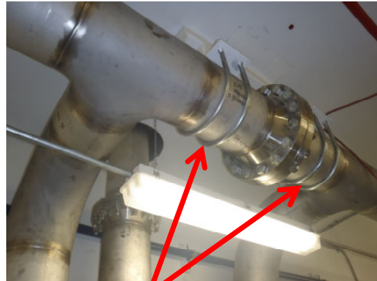
12 inch Riser Ceiling Pipe Support (PS-8)
