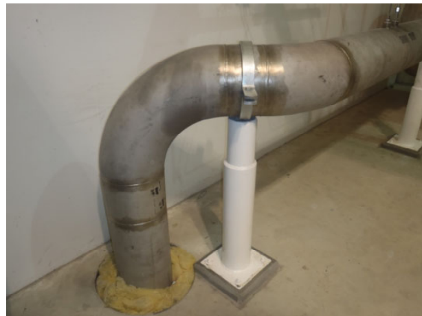
12 inch Riser Pipe Support (PS-9)
