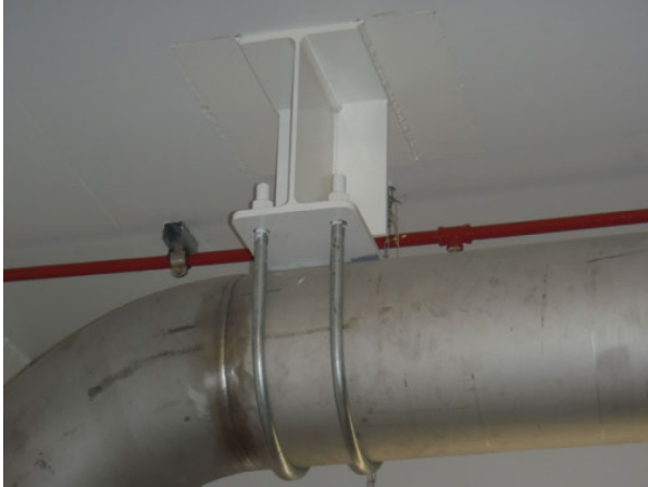
12 inch Riser Ceiling Pipe Support (PS-3)
