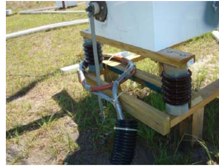
Figure 10. Two fiber loops (inside a garden hose) measuring current exiting the shunt resistor (box).
