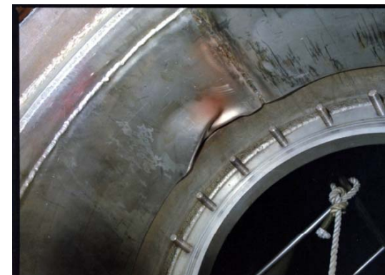
1985 Damage to Manway Liner
