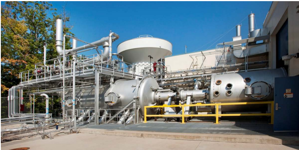
Figure 1.— Photograph of Spray Cart and Test Capsule of ACS Facility
