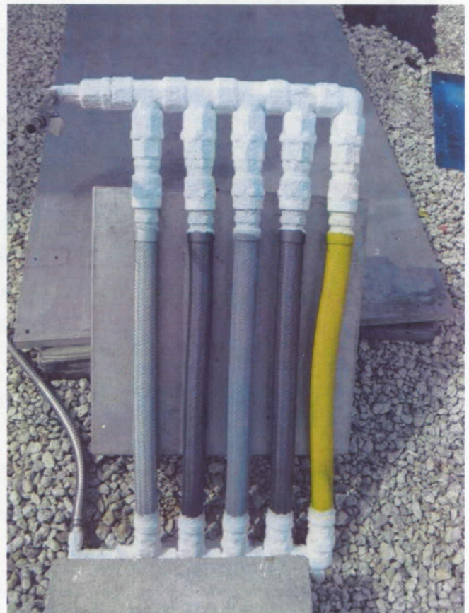
FIGURE 2 – Flex hose manifold.
