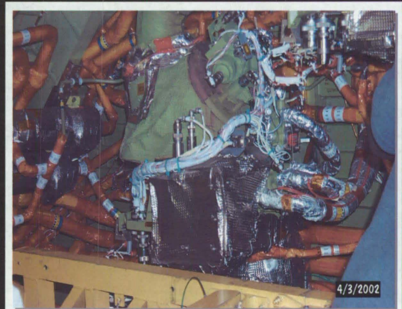
Example: Space Shuttle Auxiliary Power Unit
