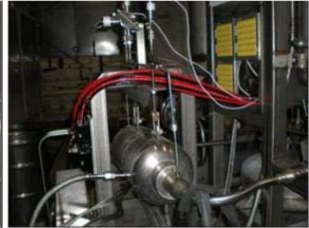
Power Cable path to core
