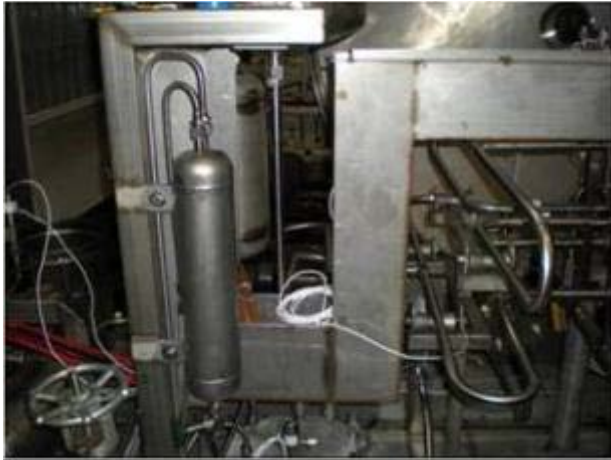
Cable tray providing protection from heat/NaK
