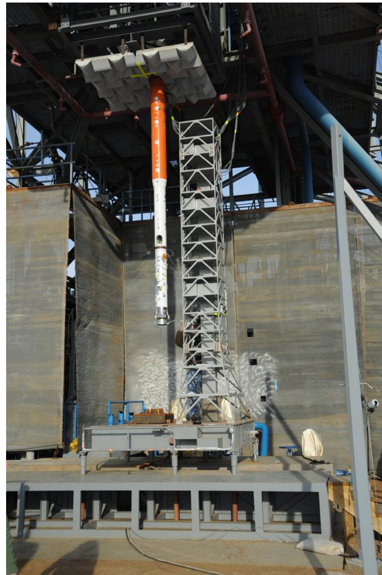
Complete Tower for VERT4-17 Elevated 5 ft and drifted
