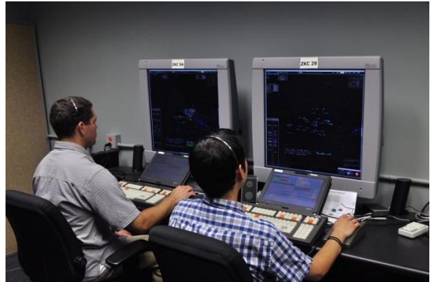
Figure 4. Air traffic controller station
