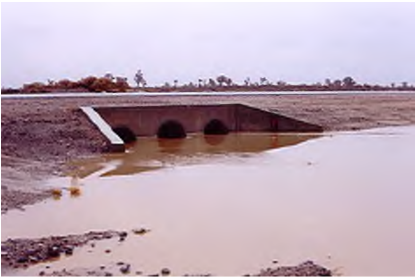
Drainage from Buckhorn at Lancaster Blvd, February 2003 (Miller et al. , 2009)
