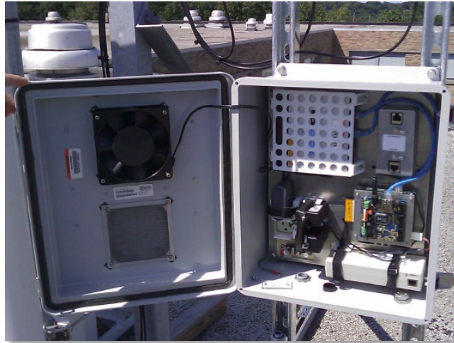
Figure 10.—Electronics equipment supporting prototype fixed subscriber stations during testing.
