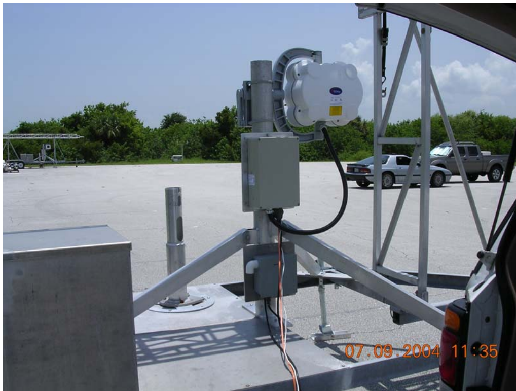
Figure 2-20 Pole Mount with OTU, Connection Box & Power Supply Box
