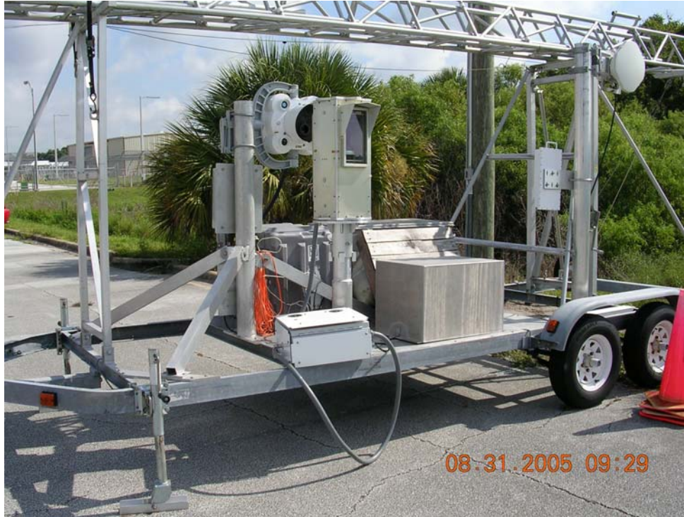
Figure 2-9 AirFiber #1 On Trailer #1 in EDL Parking Lot
