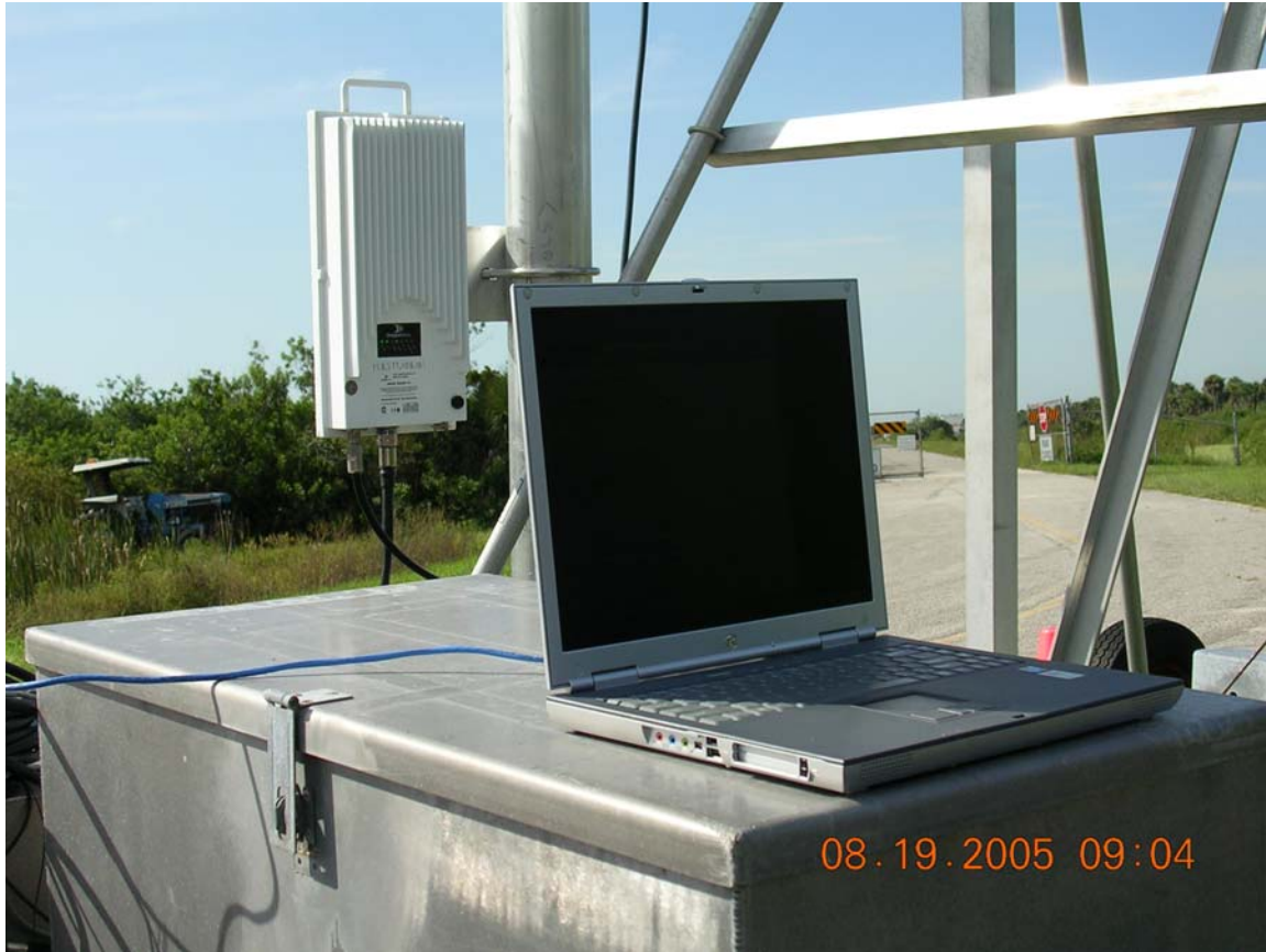
Figure 3-7 Laptop connected to the AirPair 100 Modem
