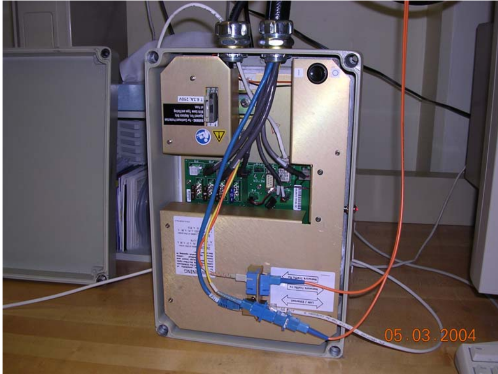
Figure 2-19 SONAbeam Junction Box Open
